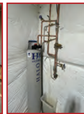
WATER PURIFICATION SYSTEMS
