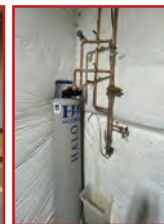
WATER PURIFICATION SYSTEMS
